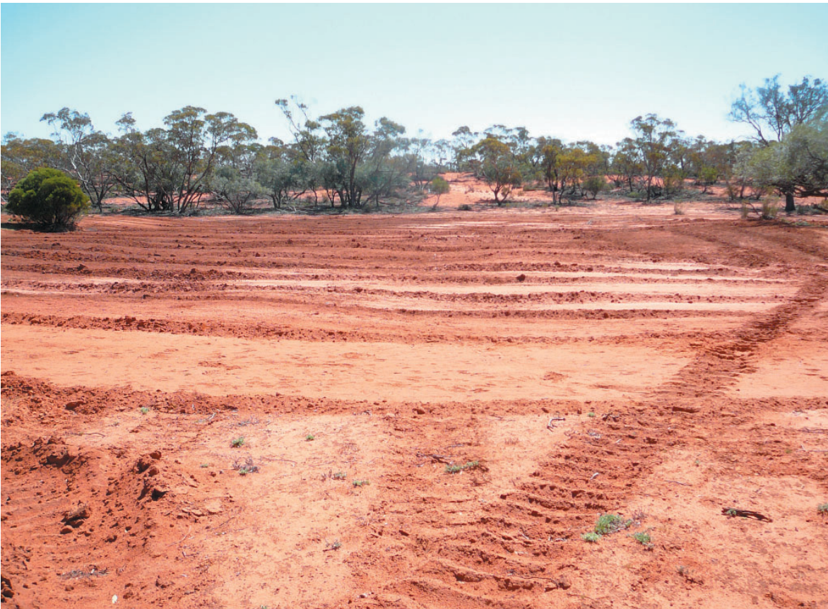
Figure 10. Functional and landscaped ground tanks
